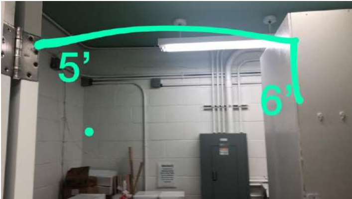
Server room location.
